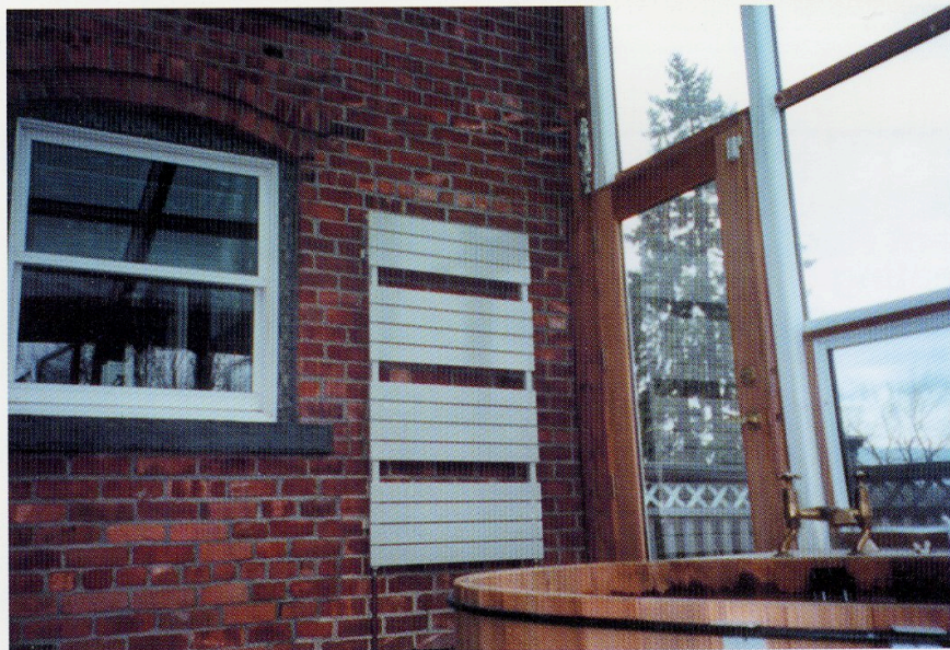
Runtal towelwarmer provides supplemental heat in the Solarium/Hot tub room.
