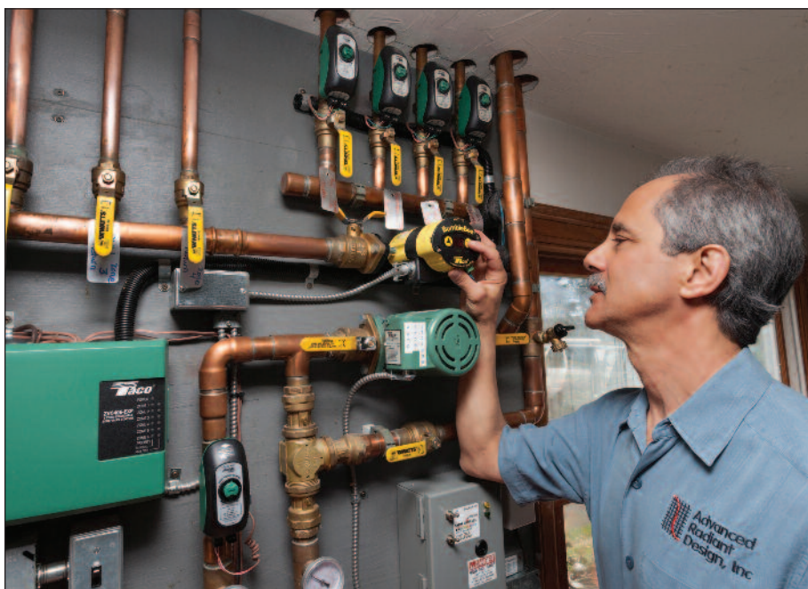
John Abularrage checks the function of a Taco Bumble Bee circulator at another biofuel job just a few miles down the road from the Triform facility.
