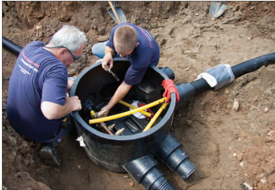
Mike Cahill, job foreman and shop manager, and Bob Witte, assistant mechanic, make Watts Radiant R-Flex supply and return connections inside an R-Flex distribution vault.
