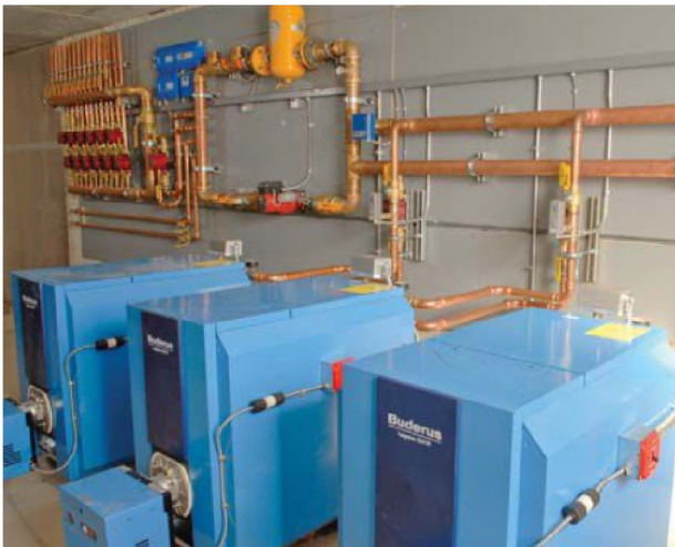
Oil-fired boilers are staged, reset, and rotated with a boiler staging control.
