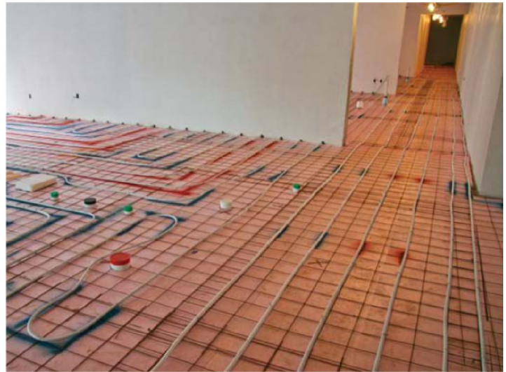
After the building was constructed, more than 15 miles of tubing in different sizes was passed through hundreds of sleeves in the walls.
