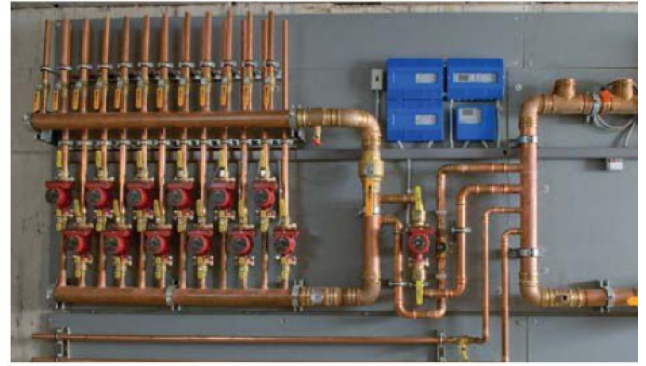
One of the two injection mixing systems feeds 12 of the 18 zones.
