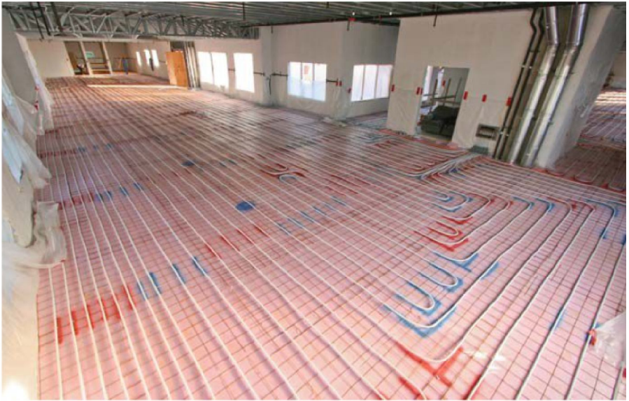
The sheer size and shape of the building with its long narrow wings and many rooms – all divided by poured concrete partition walls – presented a challenge.
