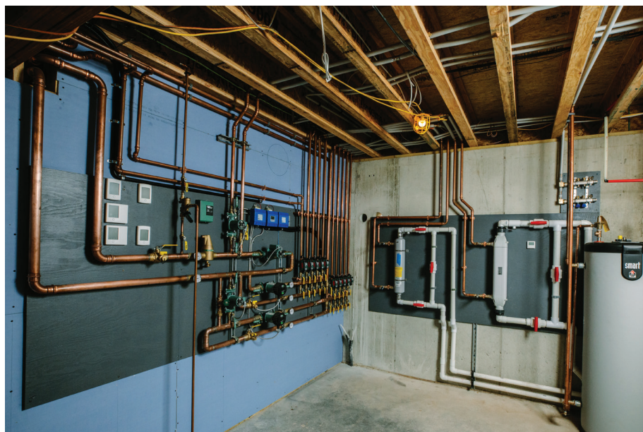
A completed mechanical space at a jobsite.
