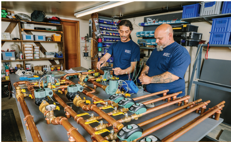
Alan Cruz, lead mechanic, and Justin Wolfe, lead technician, wire tekmar controls into a hydronic panel.
